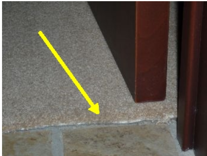
lifting at seams / edge in Bedroom #2
