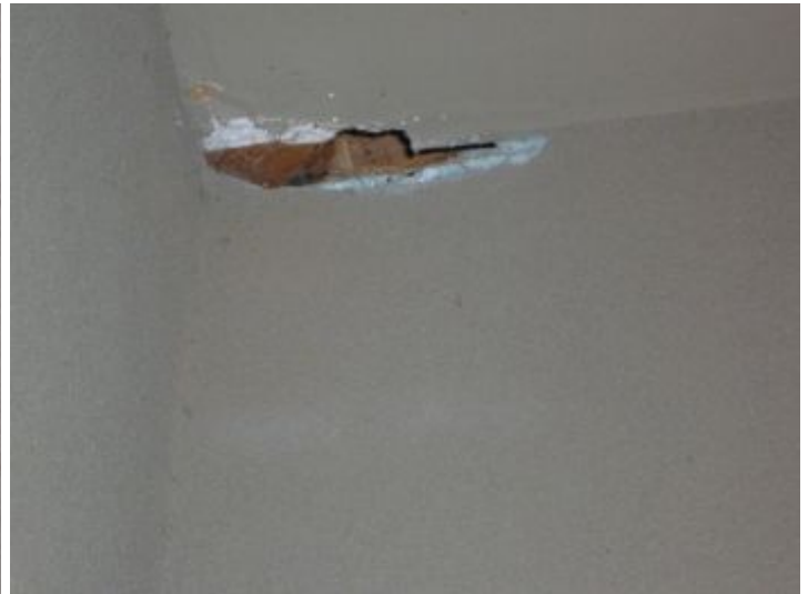
recommend sealing holes & gaps
