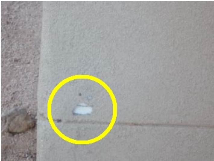
recommend sealing holes & gaps
