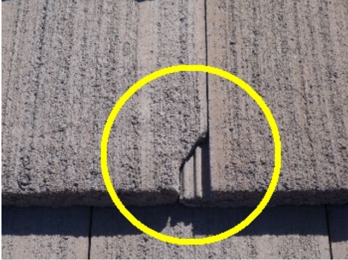
cracked tiles / broken tiles
