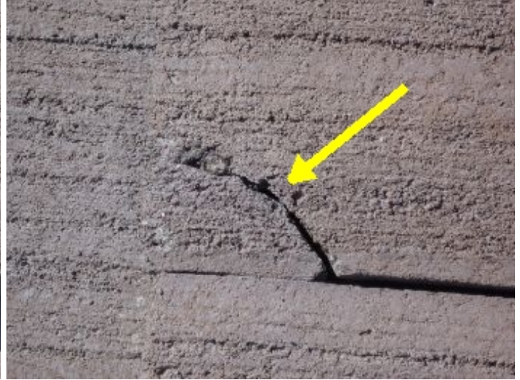
cracked tiles / broken tiles
