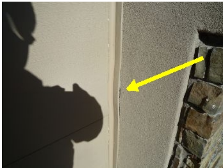
damaged weather stripping
