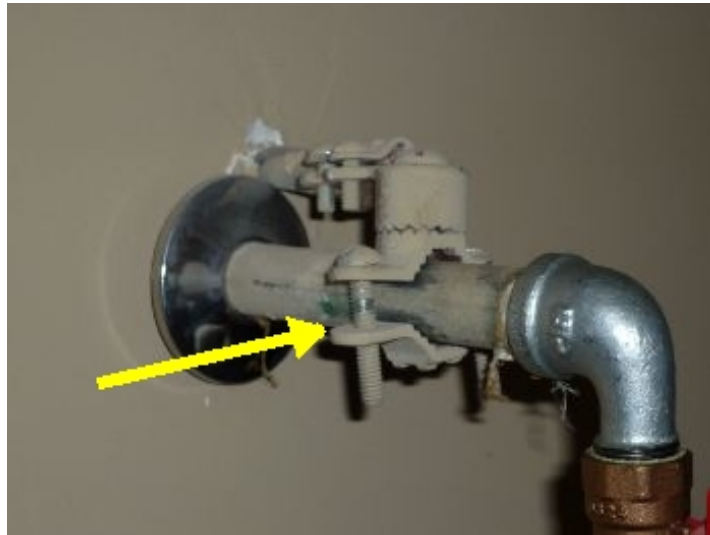
Grounding system has loose clamp
